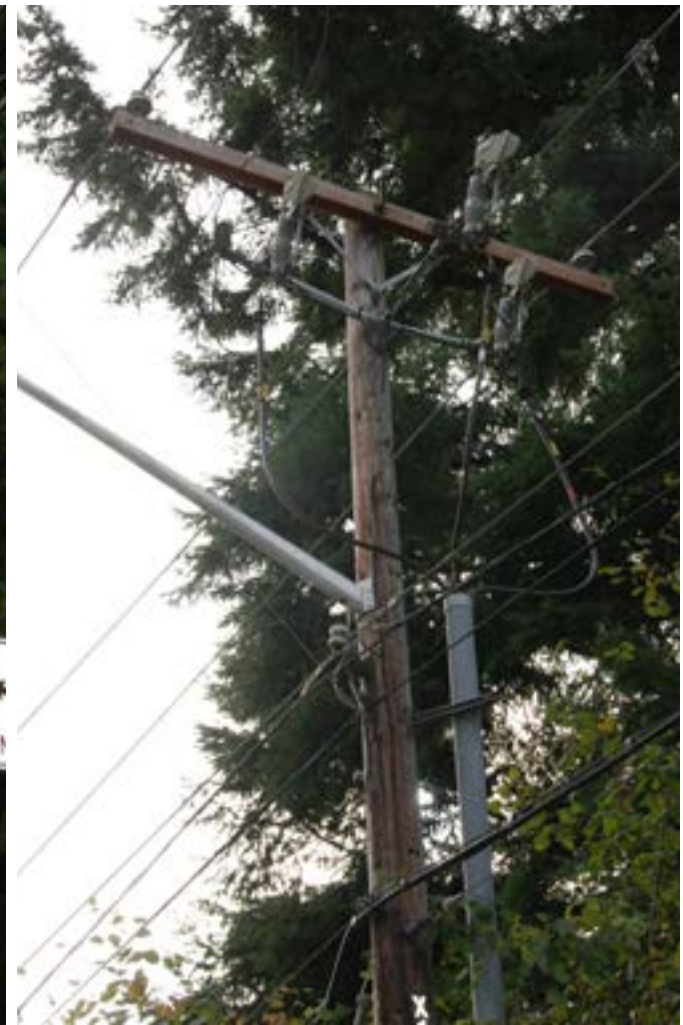
Three Phase Distribution with Three Phase Underground Distribution Termination (where underground cable system connects to the overhead system)
