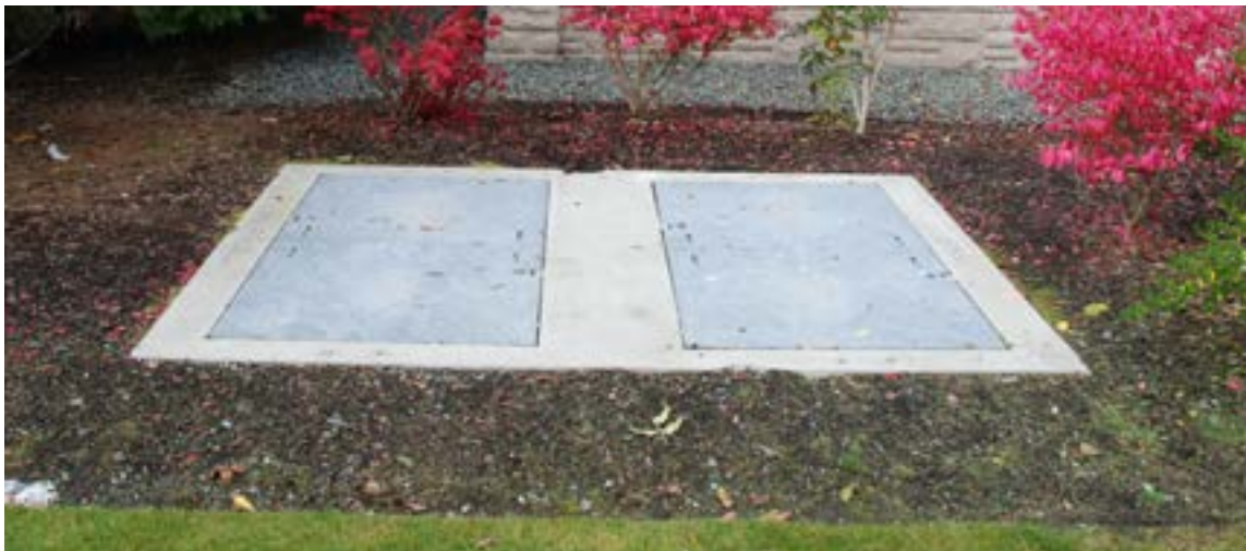
Typical Underground Distribution Vista Switch Vault (8' X 9') (the switch equipment sits completely within the vault)
