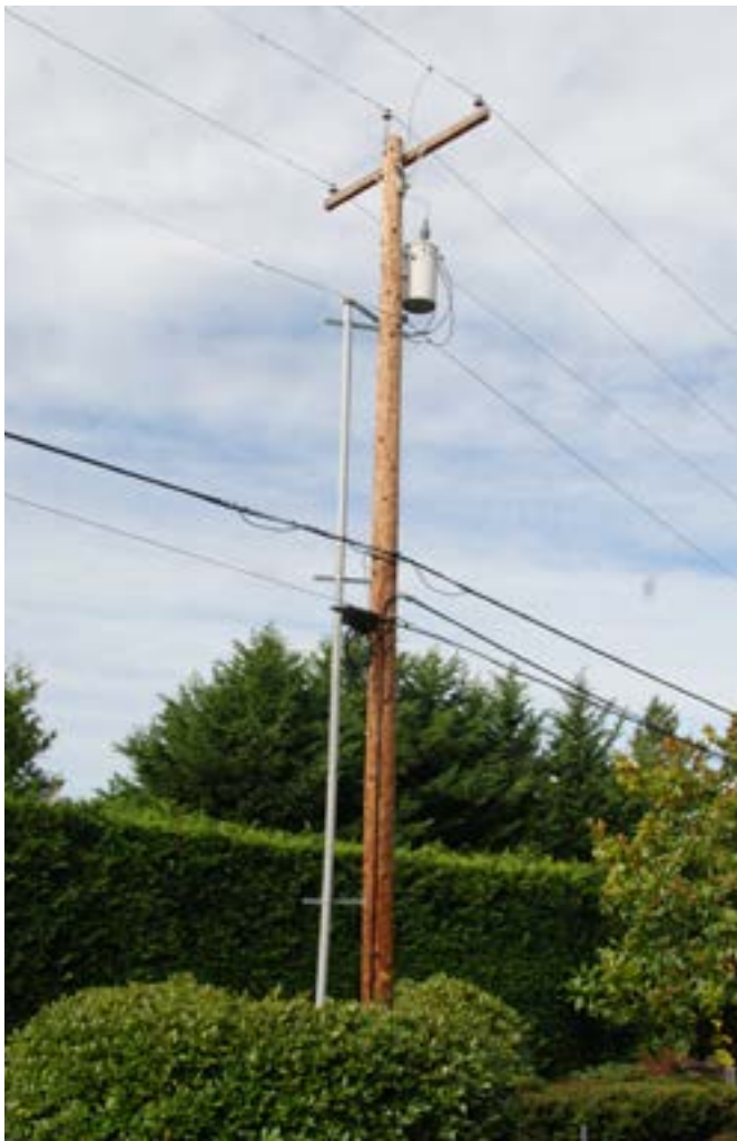
Typical Three Phase Distribution on Cross-arm (with single phase transformer and underground service connection)
