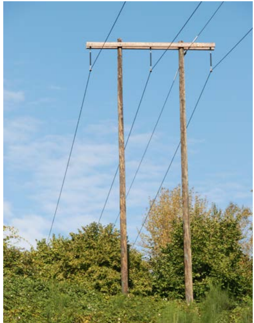
Typical 115kV Transmission H-Frame Structure
