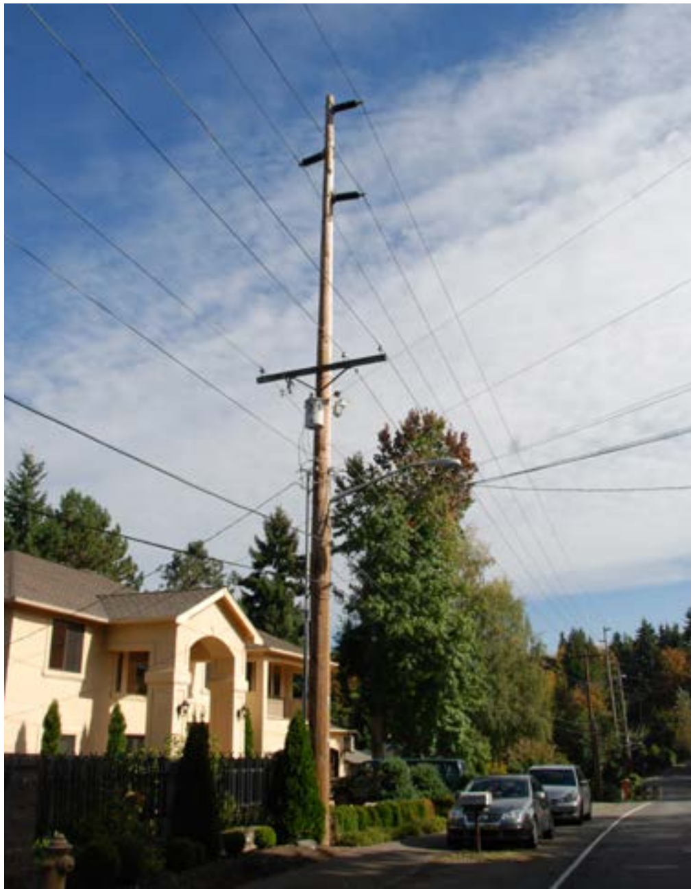
Typical 115kV Transmission Pole HPA with Distribution Under-build
