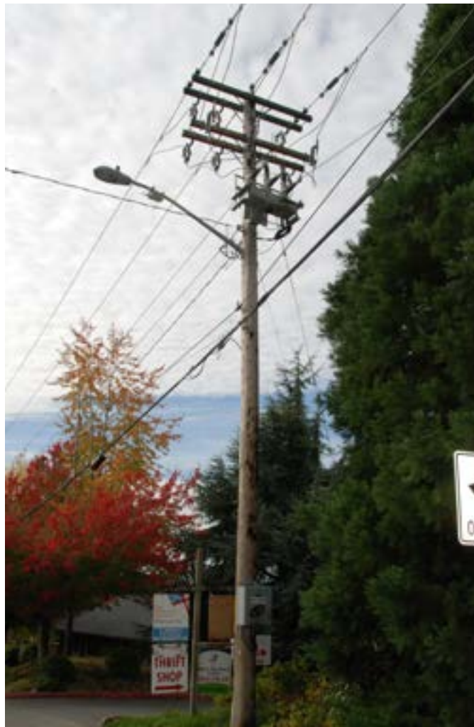
Three Phase Distribution with Recloser
