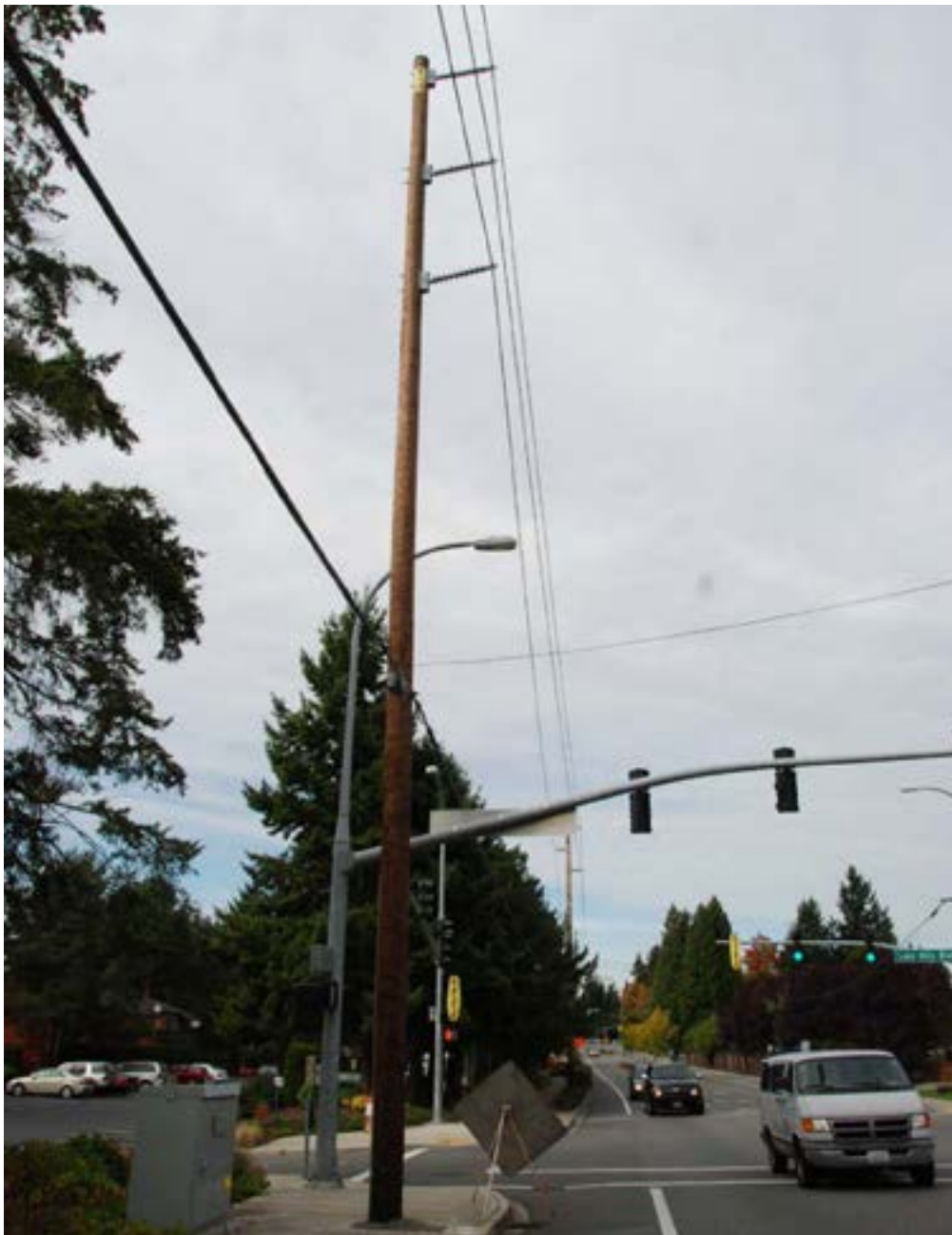
Typical 115kV Transmission Pole HPD (horizontal post directional)
