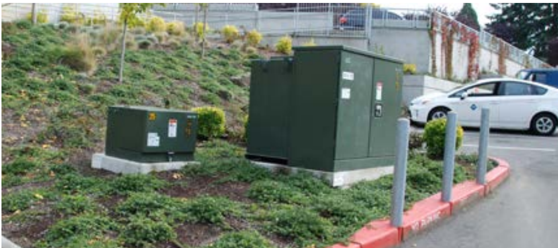
Three phase pad-mount transformers often serve a single commercial customer (but may serve multiple customers) and may be pair with single phase transformers in response to particular service needs
