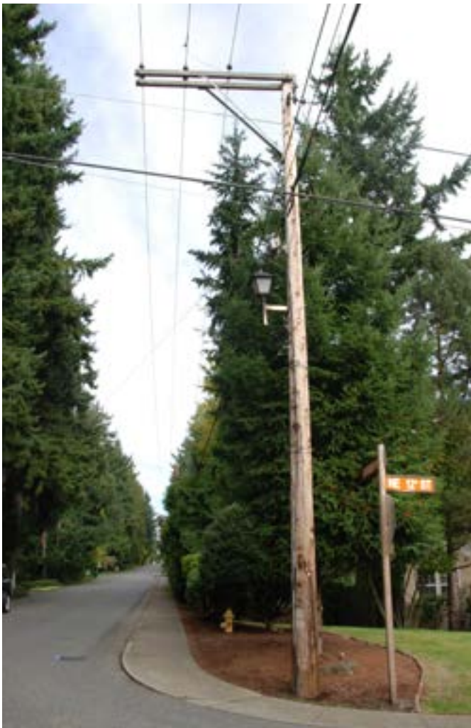
Three Phase Distribution on Wing-arm
