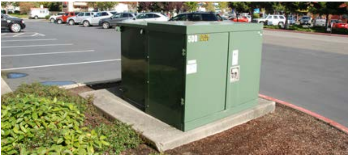
Typical Underground Distribution Three Phase Pad-mount Transformer (5' X 5' X 5' typical but can vary by transformer output rating)
