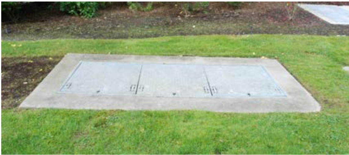
Typical Underground Distribution Feeder Cable Pull Vault (11' X 7')
