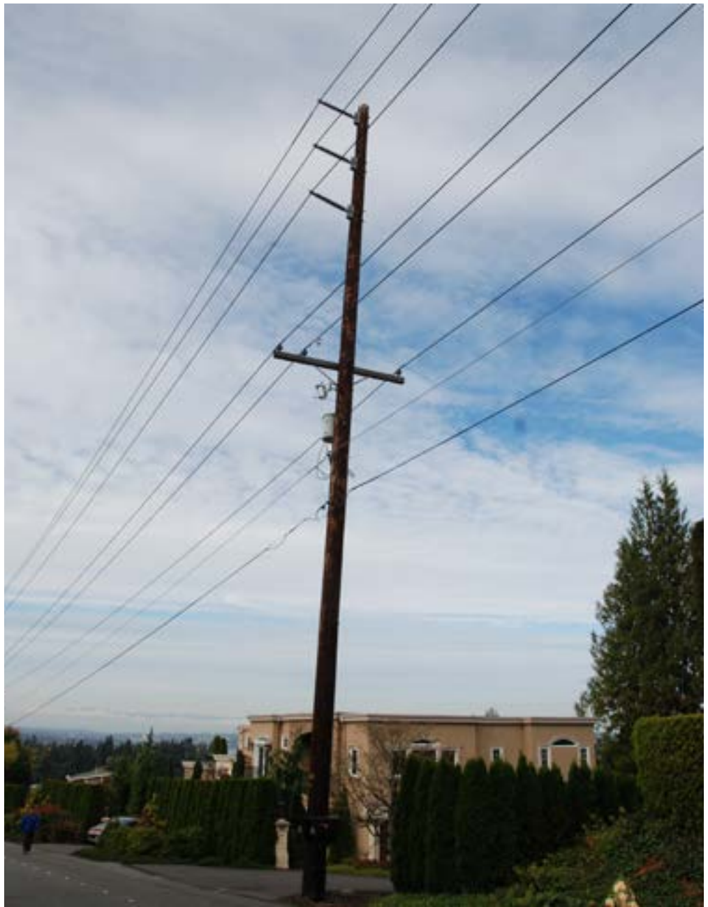
Typical 115kV Transmission Pole HPD with Distribution Under-build
