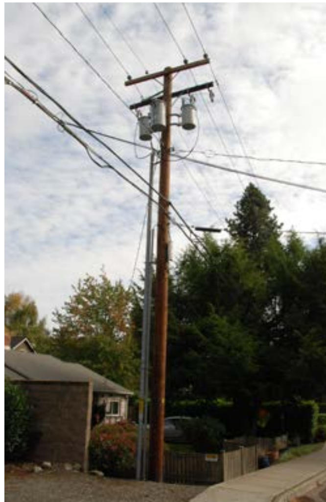
Typical Three Phase Distribution with Three Phase Transformer Bank (with underground service connections)
