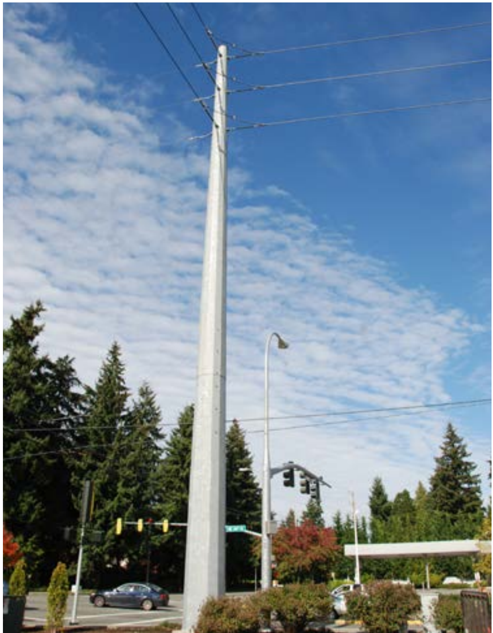
Typical 115kV Transmission Pole Steel
