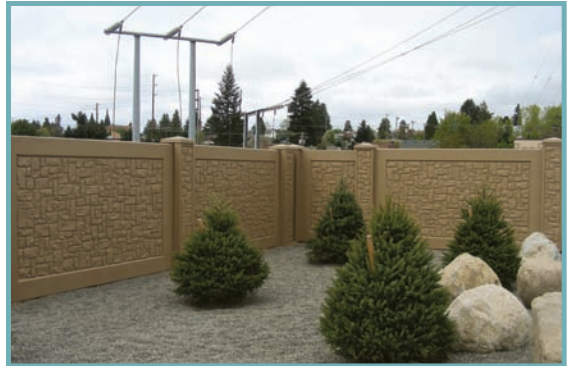
Upgraded Bremerton substation and surrounding landscape with decorative fence.
